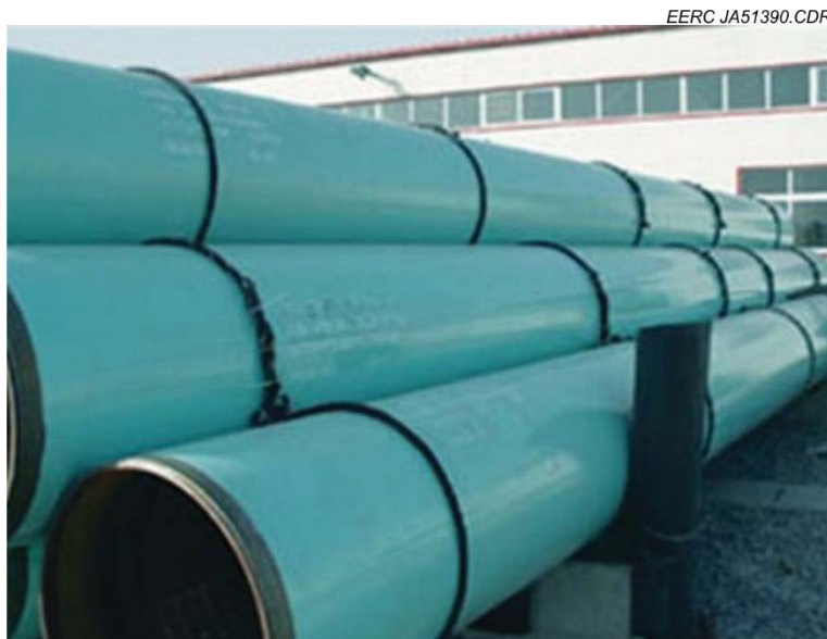
Figure E-6. Epoxy-coated steel pipeline.
